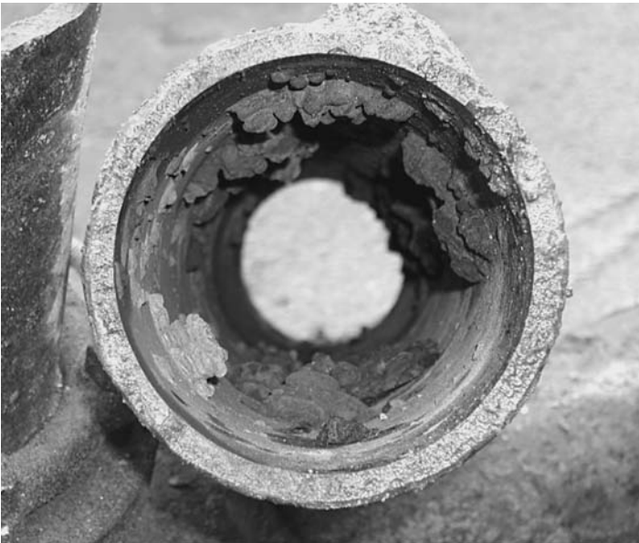
FIGURE 8.1 Tubercles in a small diameter water pipe. (Courtesy of Public Works and Services, City of Ottawa)
