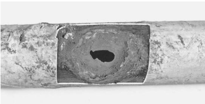
FIGURE 13.34 Pipeline perforated by a large fault current. (Courtesy of MACAW's Pipeline Defects, published by Yellow Pencil Marketing Co)
