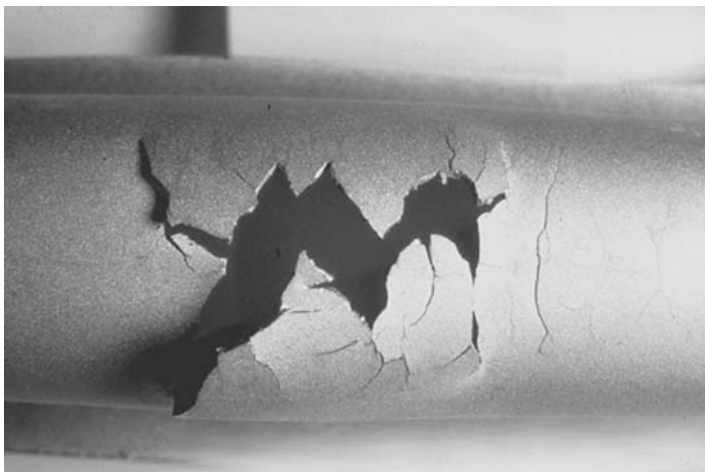
FIGURE 8.16 Type 321 stainless steel expansion joint in 2.8 MPa (400 psi) steam service cracked from caustic carryover in the steam. ( Corrosion Basics: An Introduction , 2nd edn., NACE International, by permission)
