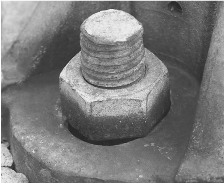
FIGURE 9.6 Galvanized bolting assembly after 10 years of exposure to a deicing salt environment.
