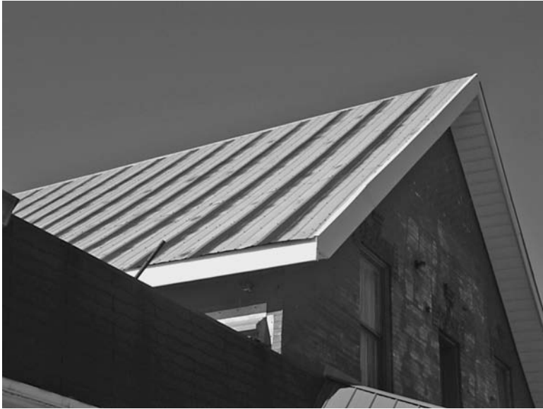
FIGURE 9.1 Rusting galvanized roof with regular bands of rust.
