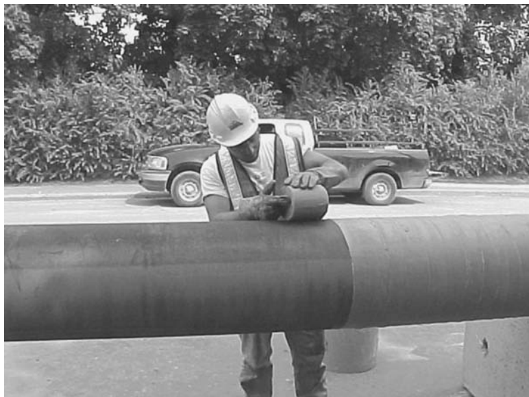
FIGURE 10.6 Wrapping a water main pipe with adhesive tape to provide a barrier against soil corrosion. (Courtesy of Drinking Water Services, City of Ottawa)
