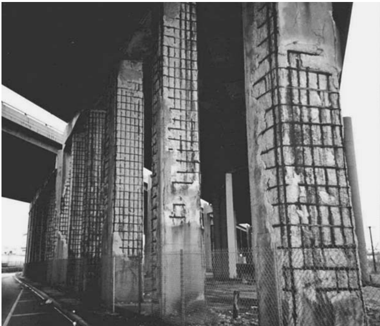
FIGURE 13.19 Corrosion ravaged columns of a highway bridge in Illinois. (Courtesy of Vector Corrosion Technologies)
