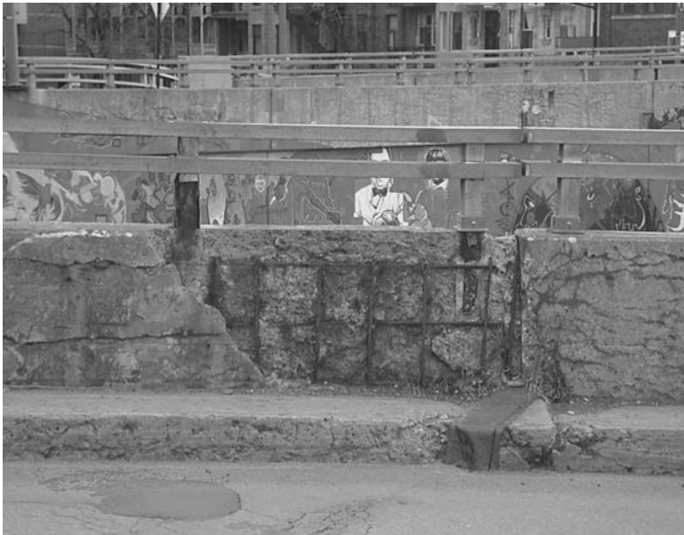
FIGURE 9.15 Reinforced concrete spalling off due to corrosion of steel rebar.
