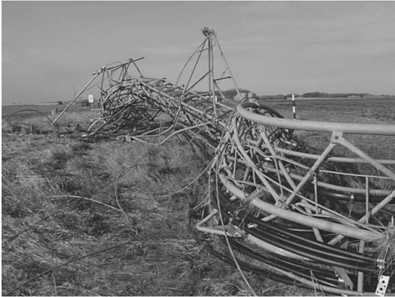
FIGURE 7.16 Mangled communication tower fallen due to loss of the anchor shown in Fig. 7.15. (Courtesy of Anchor Guard)
