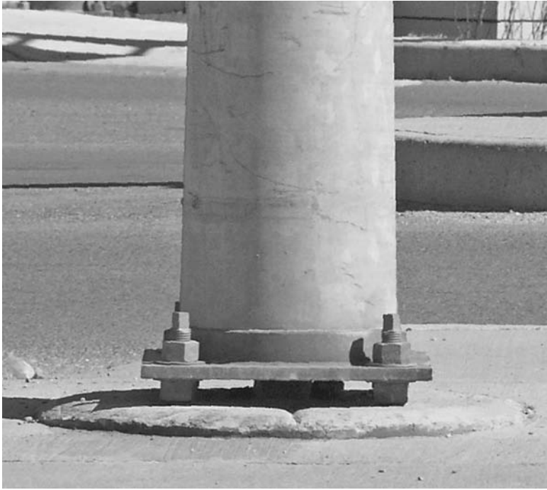
FIGURE 11.20 Lamppost galvanized steel base with a gap over the concrete to prevent crevice corrosion and pack rust.
