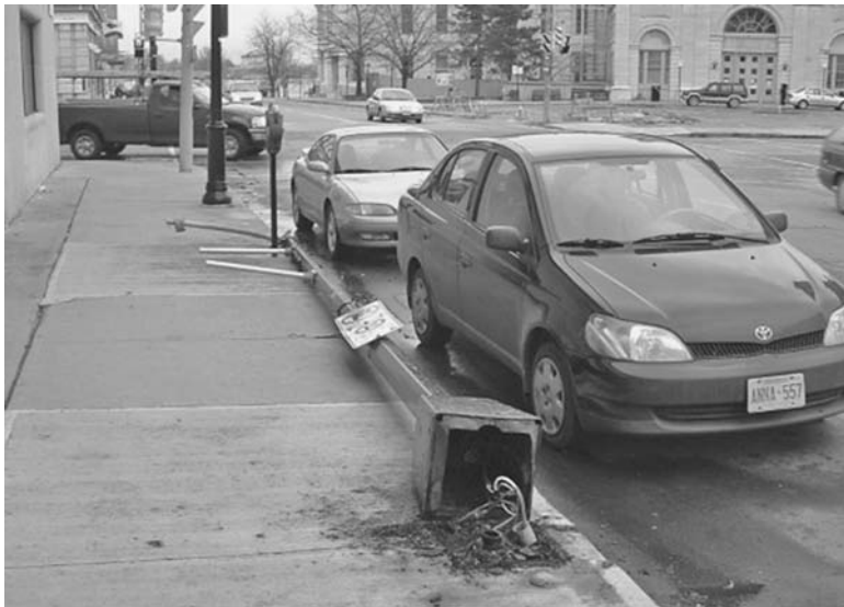
FIGURE 11.17 City lamppost fallen due to corrosion of its base. (Courtesy of Bruce Hector, Rust Check Kingston)
