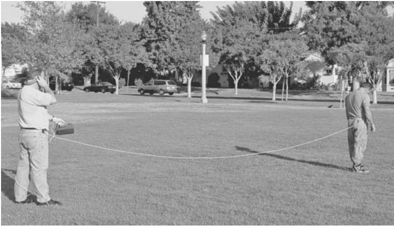
FIGURE 13.39 Pipeline CP fault testing with Pearson-type detector. (Photo courtesy of Tinker & Rasor)
