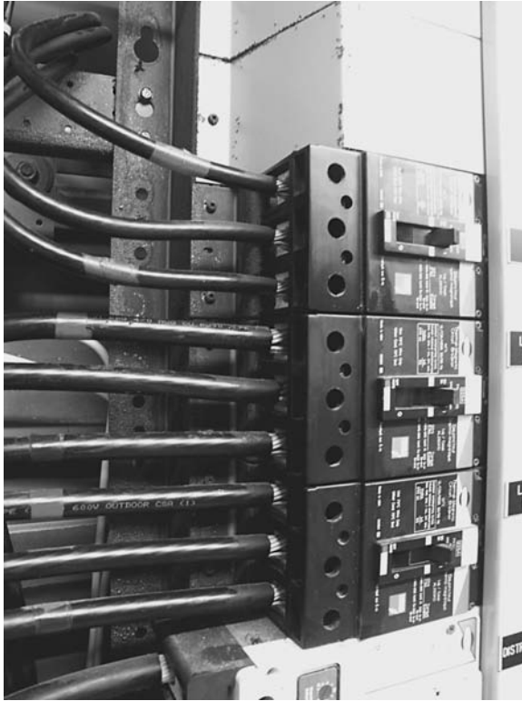
FIGURE 9.5 Electric junction box badly corroded only four years after a new residence was completed. (Courtesy of Kingston Technical Software)
