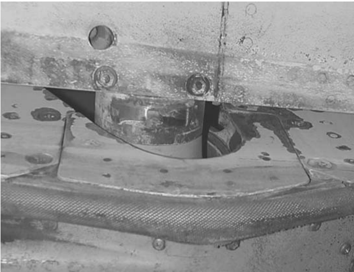
FIGURE 6.50 Fretting corrosion at the interface of two highly loaded surfaces which are not designed to move against each other. (Courtesy of Pacific Corrosion Control Corp)
