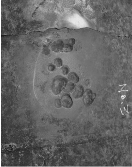
FIGURE 10.3 Typically deep, sharp-sided pits usually found under disbonded coatings or hard accumulations on a pipe surface. When disturbed the area may smell of hydrogen sulfide, a telling sign of microbial activity. (Courtesy of MACAW's Pipeline Defects, published by Yellow Pencil Marketing Co.)
