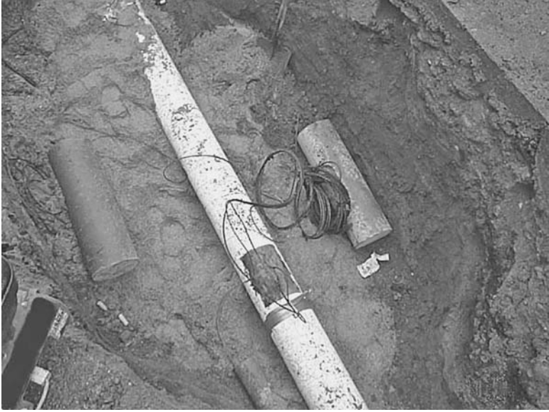
FIGURE 13.16 Ductile iron municipal watermain protected with tape wrap and sacrificial magnesium anodes. (Courtesy of Dean Rookes, West Coast Corrosion Prevention Ltd.)
