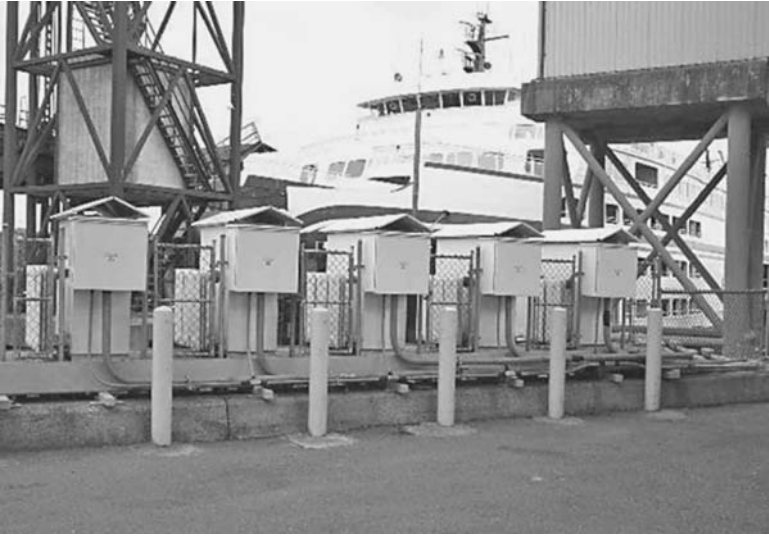
FIGURE 13.28 Five 300 ampere marine oil cooled rectifiers supported by an automatic dewatering oil spill containment pan. (Courtesy of Dean Rookes, West Coast Corrosion Prevention Ltd.)
