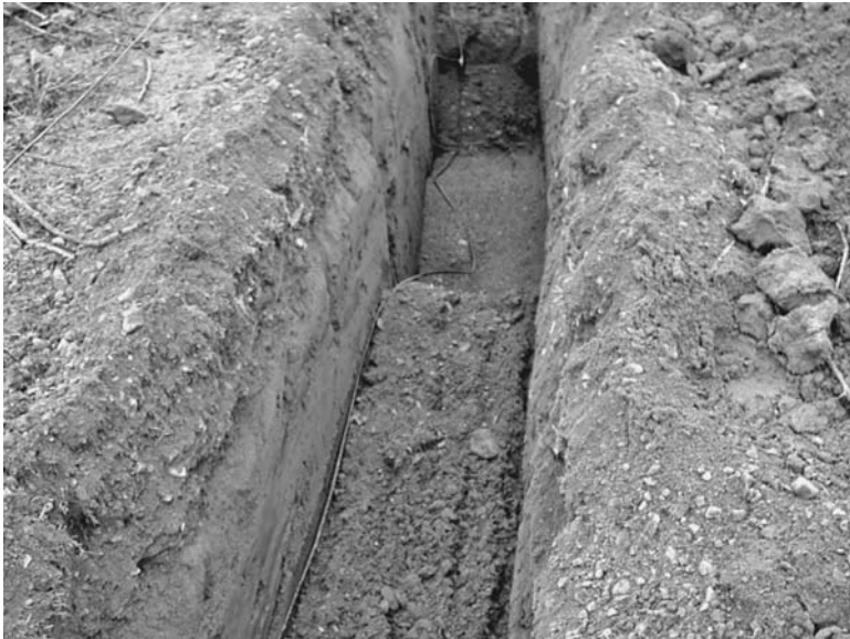
FIGURE 13.18 Conventional groundbed using petroleum coke backfill and 5 cm cast iron anodes. (Courtesy of Dean Rookes, West Coast Corrosion Prevention Ltd.)
