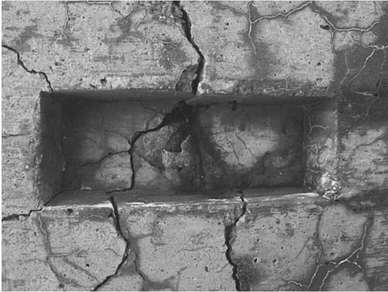
FIGURE 7.24 Cracking of concrete cover in marine environment.
