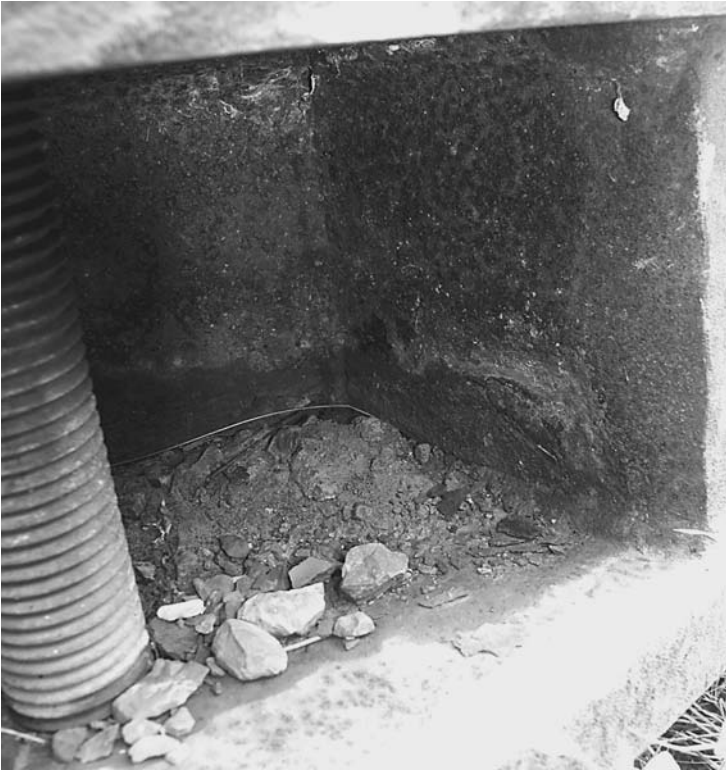
FIGURE 9.46 Pack rust developing at the base of the weathering steel highway lamppost shown in Fig. 9.45, only 15 years after its installation.
