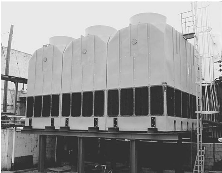
FIGURE 8.13 Three cell induced draft counterflow cooling tower made of seamless double wall polyethylene construction. (Courtesy of Delta Cooling Towers)
