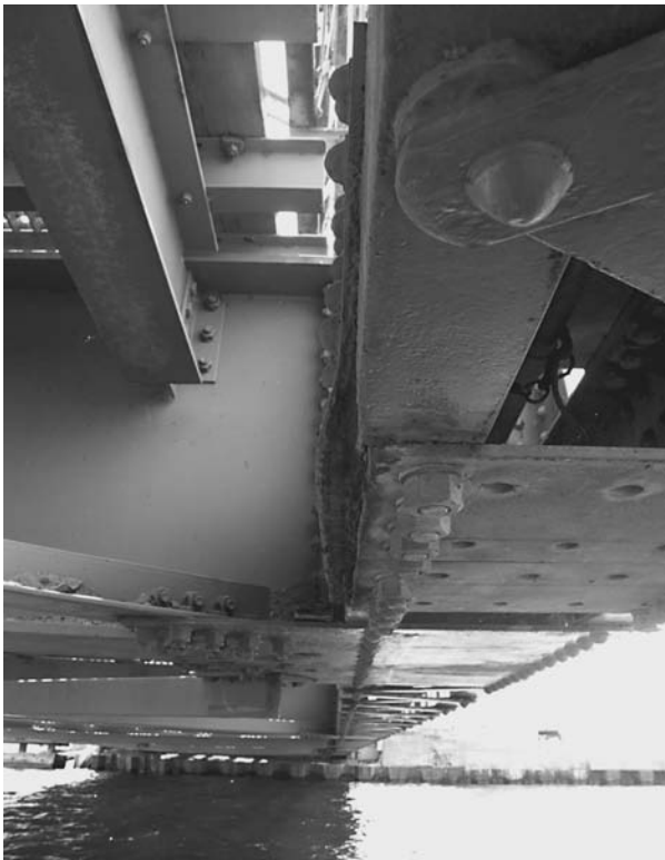
FIGURE 9.13 Pack rust under a steel bridge.
