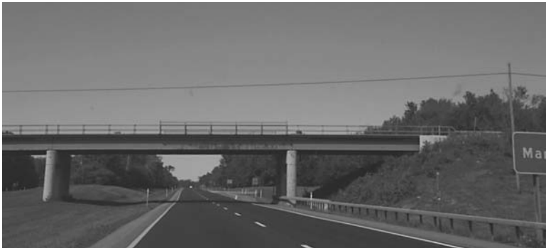
FIGURE 9.22 Corroded overpass steel bridge above the most traveled lane of a two-lane highway, a telltale symptom of deicing salt corrosion.
